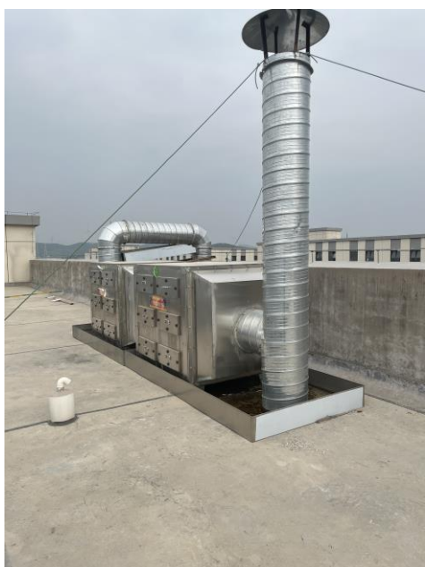
图 3-3 (a) DA001 涂布烘干废气排气筒
